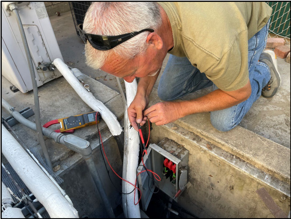
ERHS – Del Ward Running Power to the HVAC Unit in the Main Server Room
