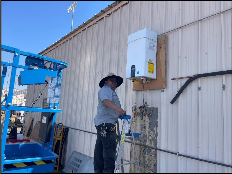
SMHS – Jesus Reyes Installing a New Water Heater at the Maintenance Shop
