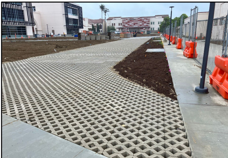
SMHS 50-Classroom Building – Fire Access Lane Pavers are Installed in the Lawn Area
