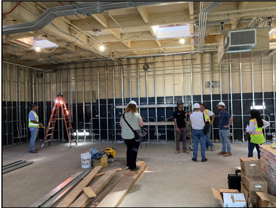
ERHS CTE Modernization – Construction Team Reviews the Progress in the Wood Shop
