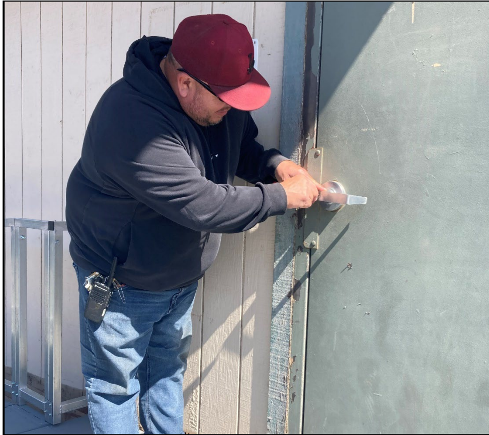
PVHS – Paul Alvarez Installs Door Key Cores for the Ten Portable Classrooms
