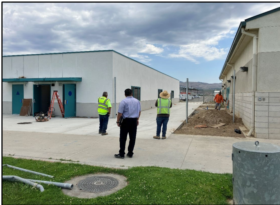
PVHS 3 New Modular Classrooms – New Fencing Separates the Classrooms from the Pool Equipment Building
