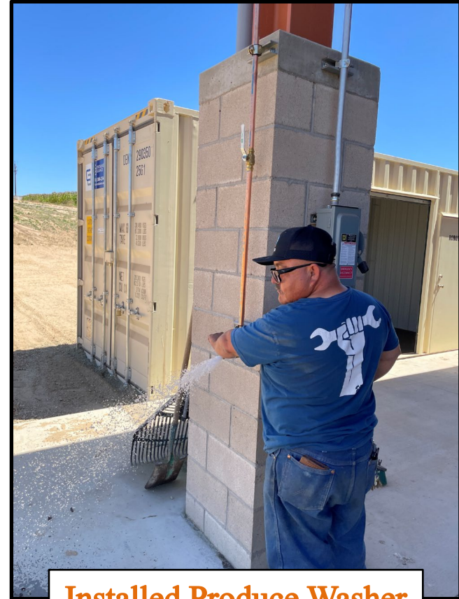
Installed Produce Washer
