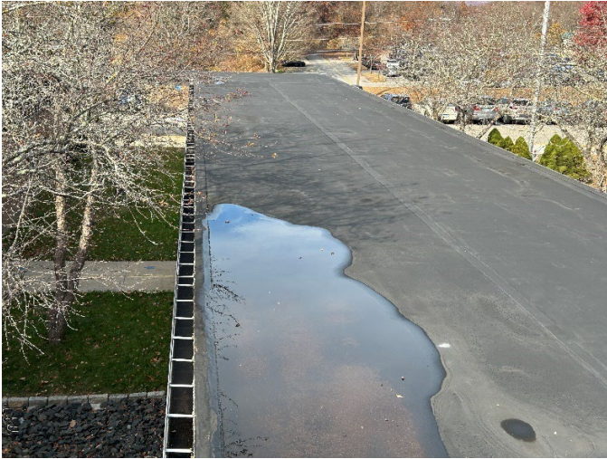
Significant ponding on low slope roofs – roof 7 (canopy)
