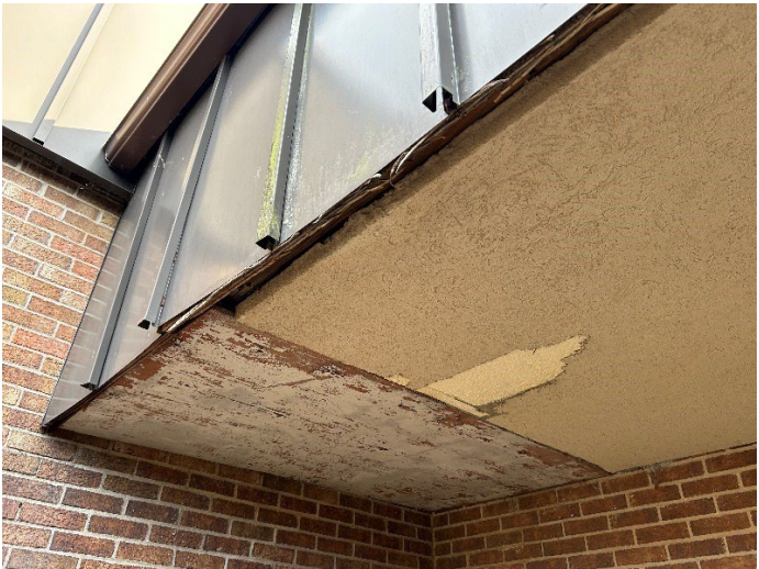
Failed metal standing seam panels & soffit
