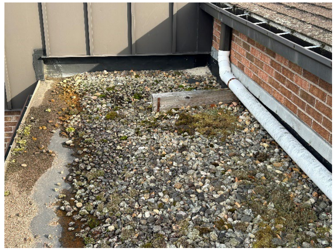
moss growth is an indication of standing water
