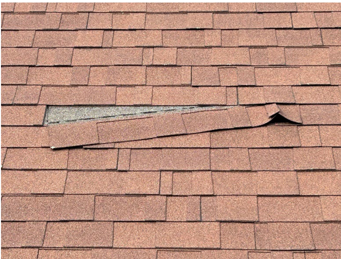
Failed Asphalt shingle at sloped roofs
