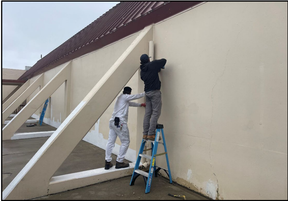
SMHS – Joel Amezcua and Tom Harbold Repairing and Painting the Exterior of the Wilson Gym
