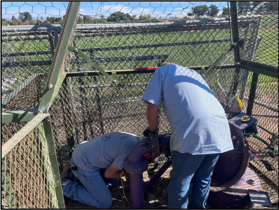
ERHS – Del Ward and Andy Freitas Pulling Wire for the VFD to the Pump House
