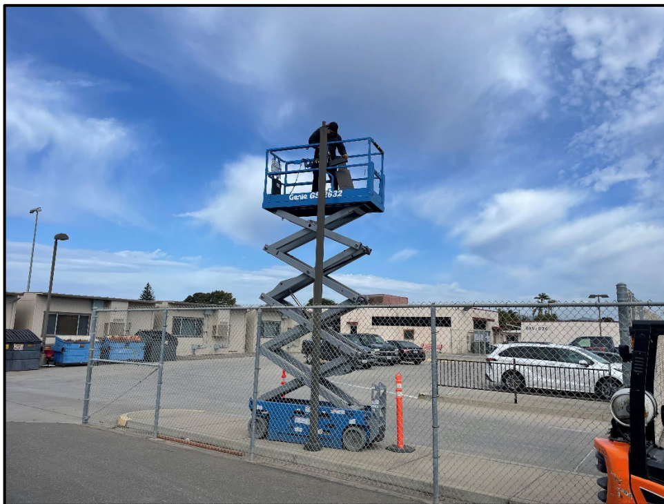
SMHS – David Velasco Repairing a Light Pole Outside of the Maintenance Shop
