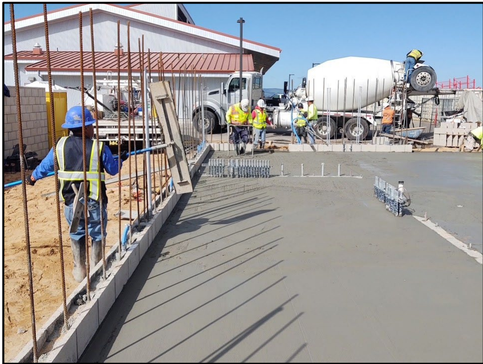
MRCTECAF M&O Building – The Concrete Floor is Finalized and Block Wall Begins
