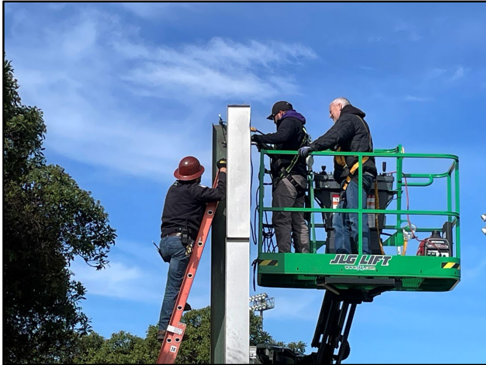
ERHS – Leo Avila, Armando Gutierrez, and Del Ward Installing the New Baseball Scoreboard
