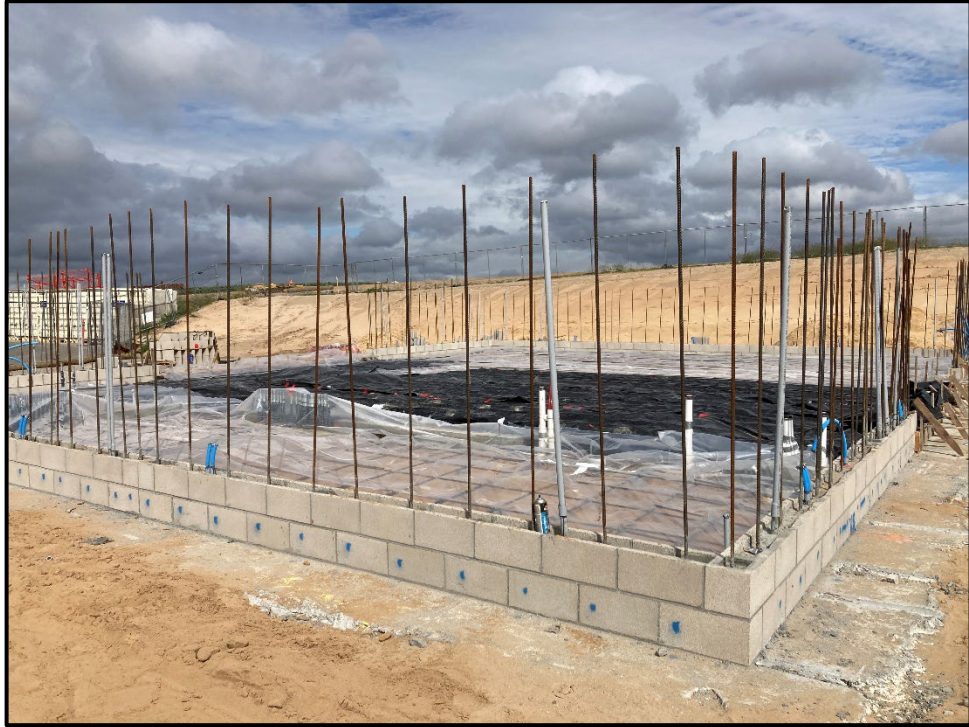
MRCTECAF M&O Building – The Concrete Floor is Finalized and Block Wall Begins
