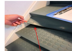
Loose stair finishes
