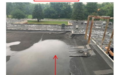
Areas of ponding.
