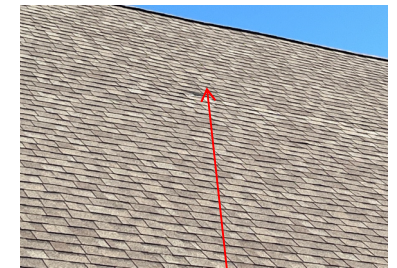
Roof shingle damage
