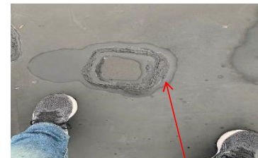
Failing roof patch joints/cement.
