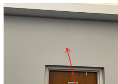
Damaged / crack in gyp. board
