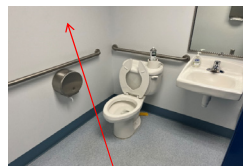
Missing vertical grab bar
