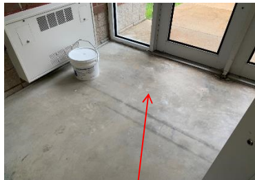
Missing walk-off carpeting at doors.
