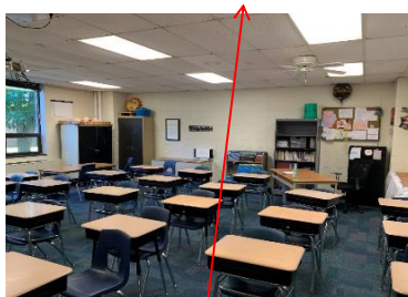
Sagging ceiling tiles.
