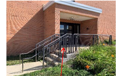
Repaint hand/guard rails.
