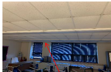
Sagging ceiling tiles.
