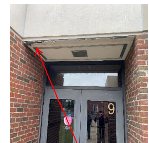
Peeling paint at entry.
