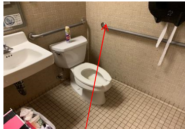
Missing vertical grab bar.
