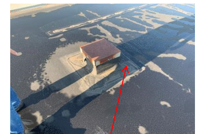
Rusting at penetration/cap.
