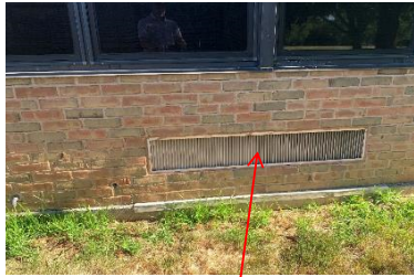
Repair / replace louver and re-seal.
