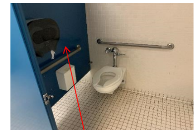
Missing vertical grab bar.
