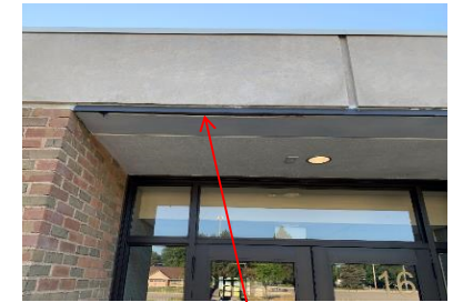
Joint opening up.
