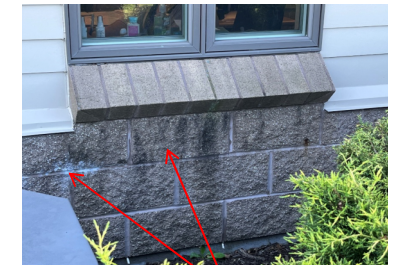
Masonry staining and efflorescence
