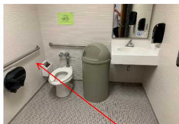
Missing vertical grab bar.
