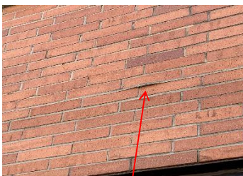
Damaged masonry and mortar joints.
