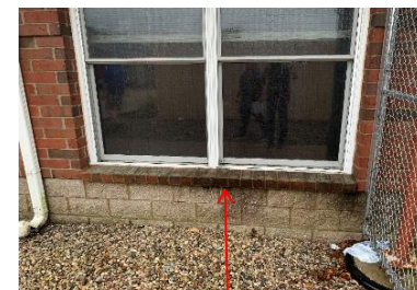
Staining at window sill.
