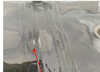
Failing roof patch
