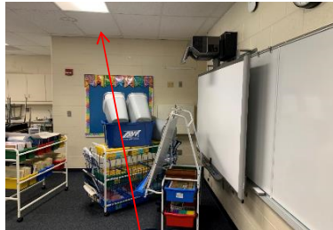
Stained ceiling tiles.
