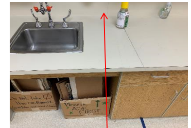
Damage to plastic laminate countertop.
