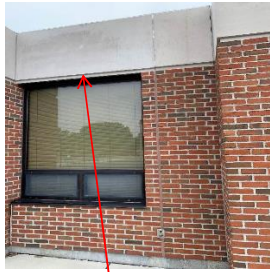
Staining on exterior wall.
