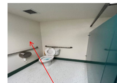
Missing vertical grab bar
