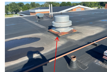
Rusting roof equipment.
