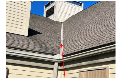
Roof flashing in poor condition
