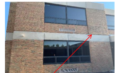
Staining on masonry.
