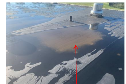
Areas of ponding.
