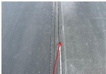
Roofing joint/seam cracking needing repair.
