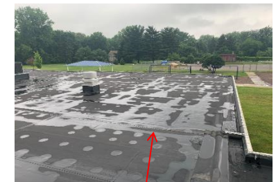
Areas of ponding.
