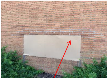
Need repairs at metal panel and masonry.
