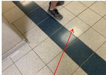
Cracks in flooring.
