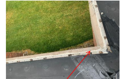
Failing roof cement/joints.
