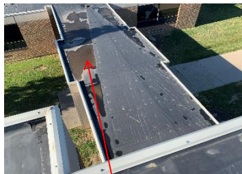
Ponding on roof.
