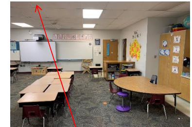
Sagging ceiling tiles.
