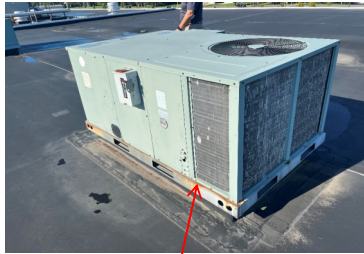
Rusting roof equipment.
