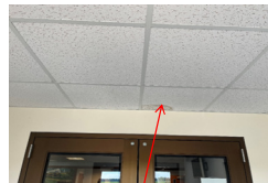
Damaged ceiling tile
