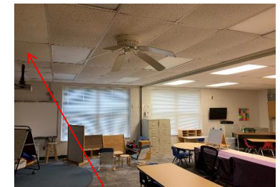
Sagging ceiling tiles.
