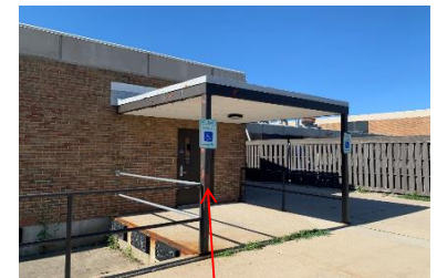
Chipping/peeling paint at entry canopy.
