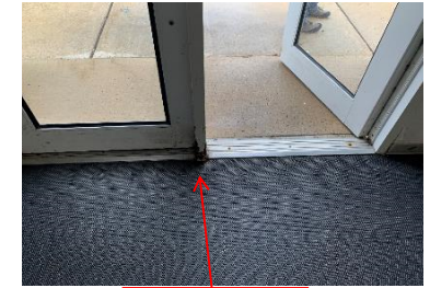
Damage at door
