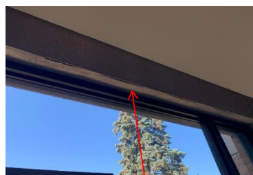
Damage at window head.
