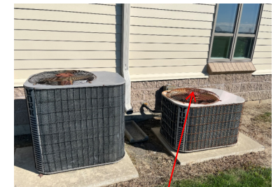
Rusting HVAC equipment
