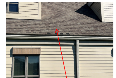
Roof shingle damage
