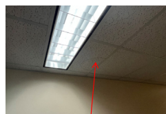
Damaged ceiling tile
