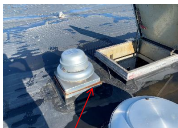
Rusting at roof vent.
