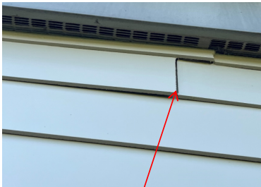
Damaged / loose siding
