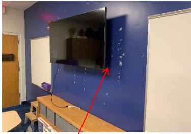
Repair / repaint walls.
