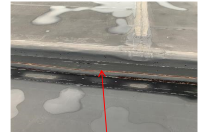
Rusting roof flashing and joint opening up.
