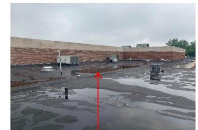
Areas of ponding.
