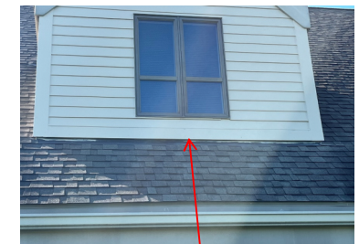
Roof flashing in poor condition
