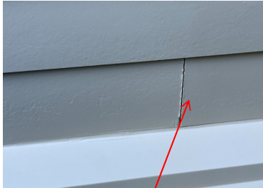
Open joint in siding
