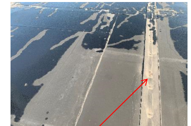
Damaged roofing material - several repairs due to
