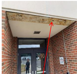
Rusting lintel at entry.
