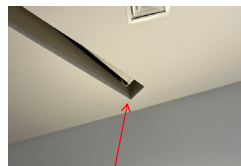
Damaged / crack in gyp.
