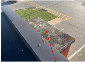
Staining on construction
