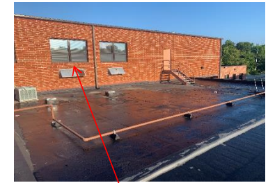
Rusting at vent.
