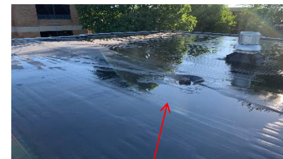
Ponding on roof.
