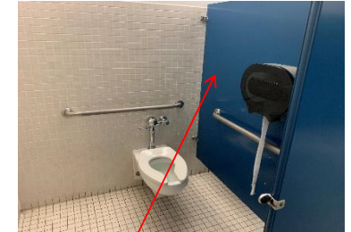
Missing vertical grab bar.
