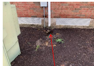
Missing downspout splash block.
