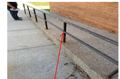
Repaint hand/guard rails.
