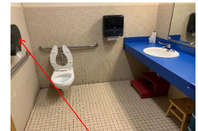
Missing vertical grab bar.
