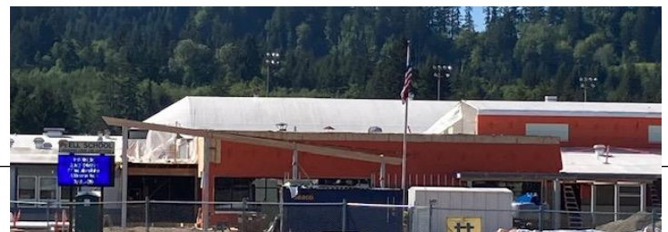
The front of the school begins to take shape. Pictured top, the middle school siding is almost complete. Bottom: the new entrance is taking shape.
