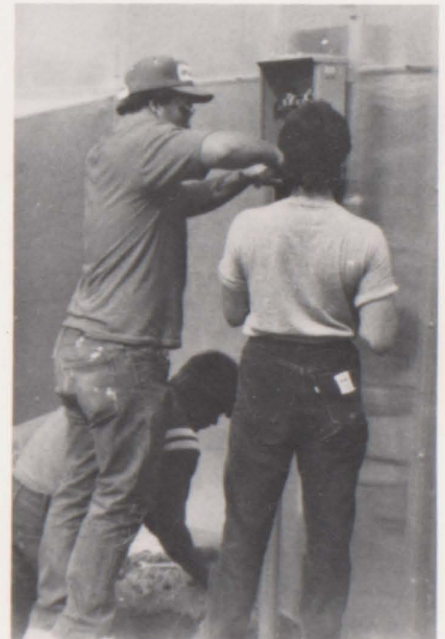
Sam Hinch, Jeff Hedgecoth, and Brenda Randolph work on the wiring in the breaker box for the greenhouse. "It was a lot of hard work, but we benefited from the experience," remarks Hedgecoth.
