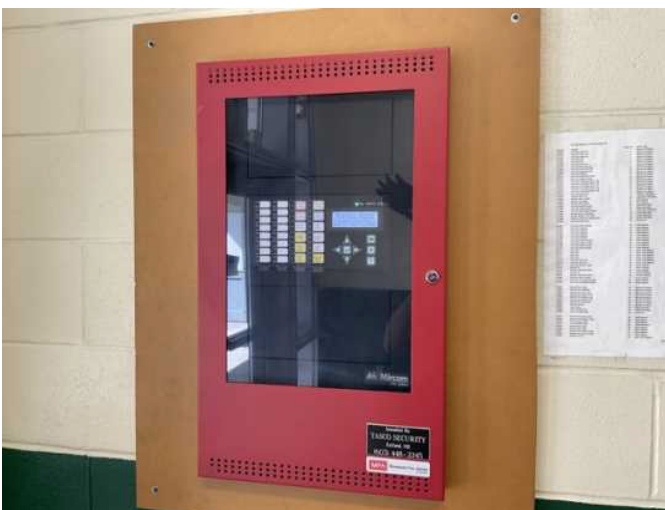
11 - FIRE ALARM PANEL
