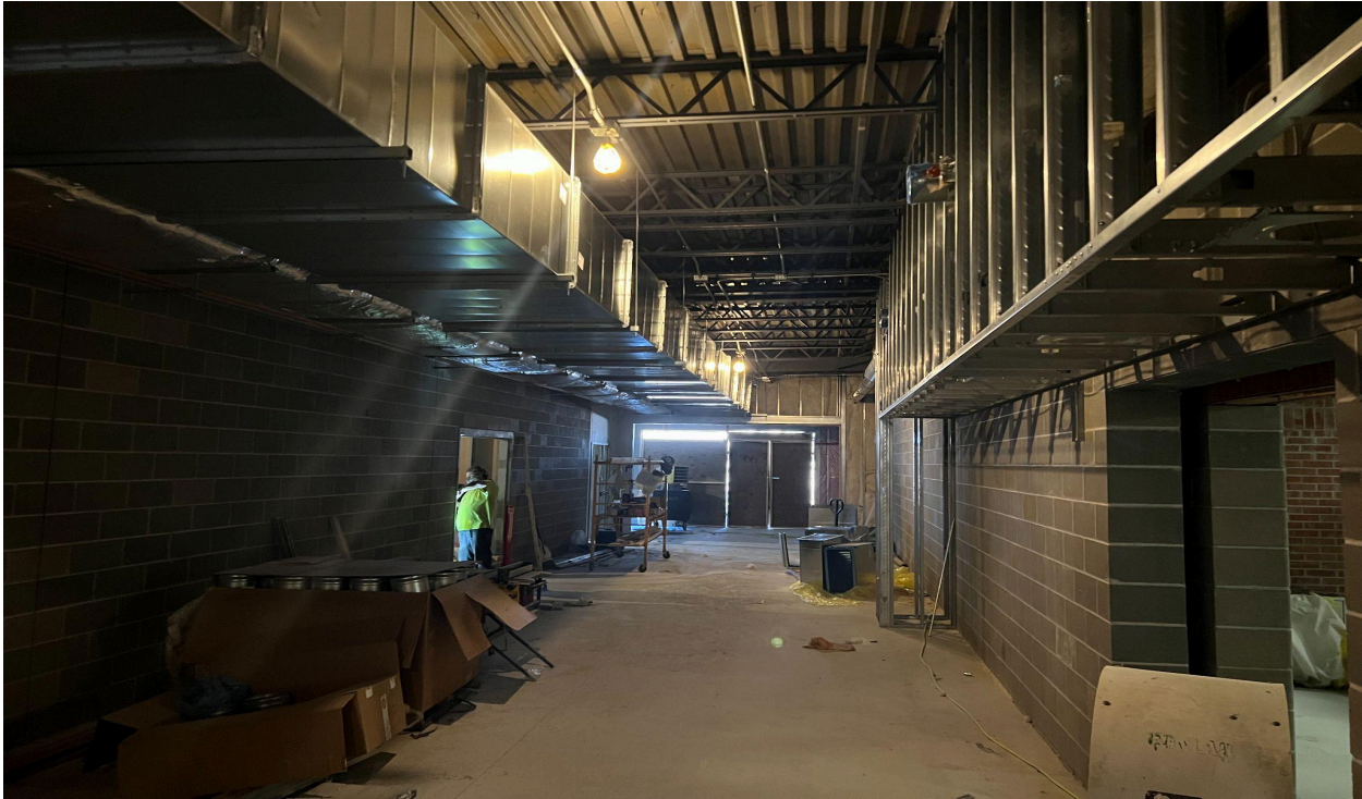
Hallway to the elementary entrance area on the north side of the new addition.
