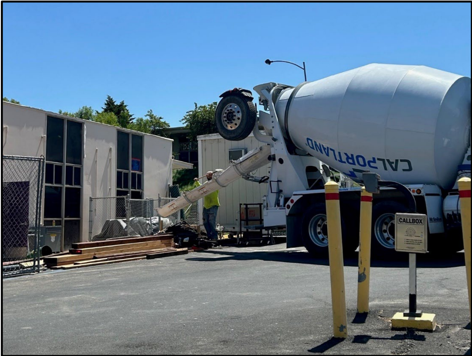
ERHS CTE Modernization – New Concrete on the West Side of the Welding Shop
