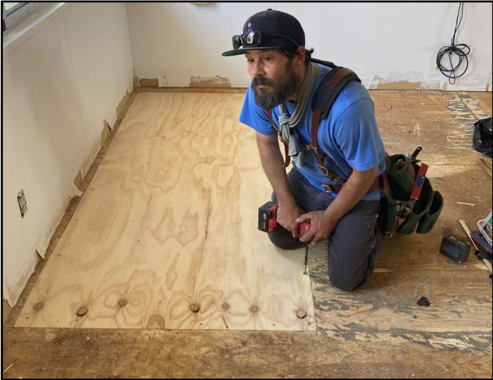
PVHS – Tom Harbold Replacing a Portable Classroom Subfloor Prior to Carpet Installation
