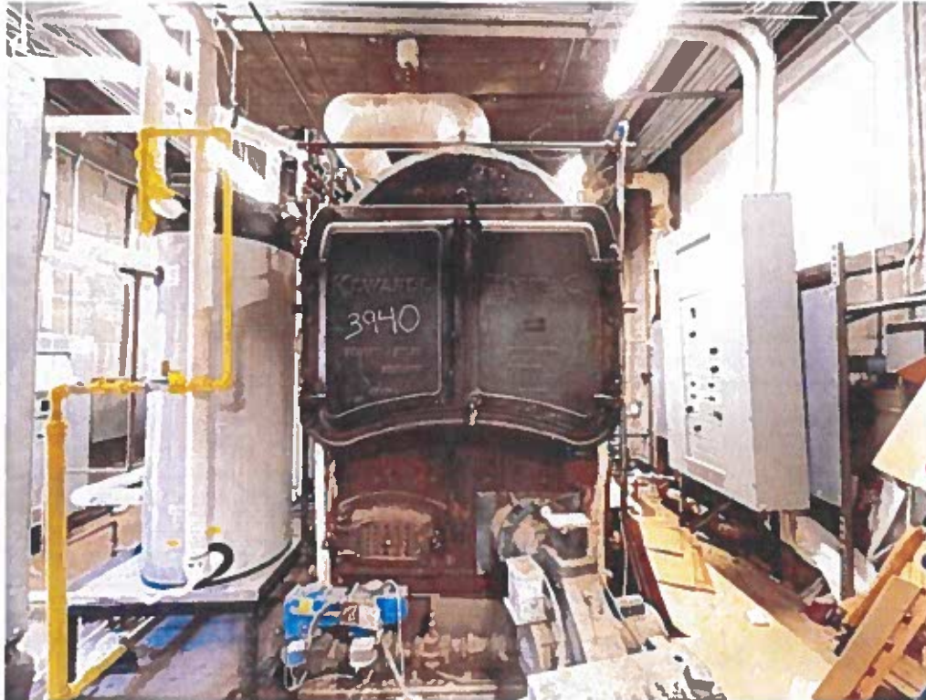
View of typical non-active 1964 boiler. 1 of 3 boilers in the original 1949-1950 structure.
