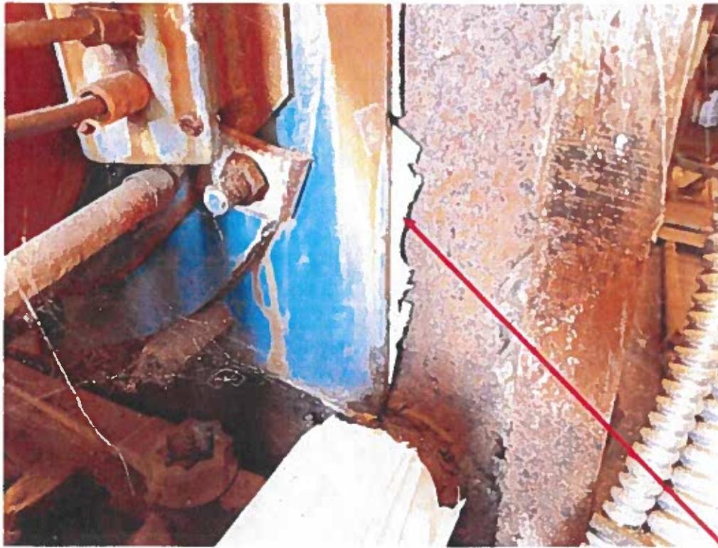
View of pressed board gasket material located on all three boilers. Friable but asbestos was non-detect in samples.
