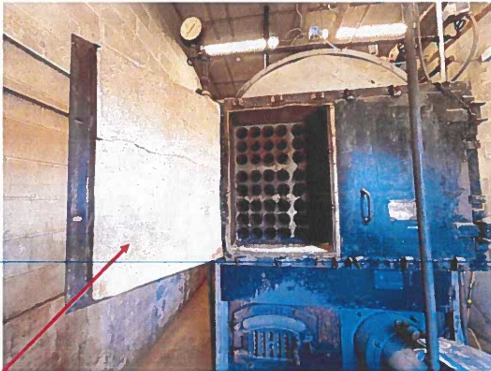
View of typical inside of door panels, friable asbestos-containing insulation.
