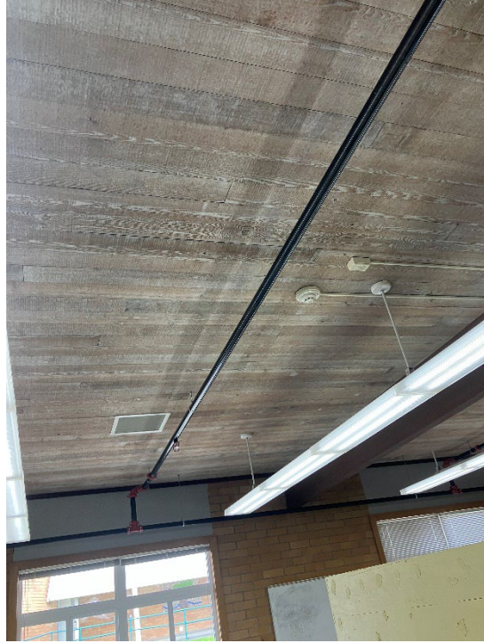
About a third of the new classroom fire sprinklers are in place.
