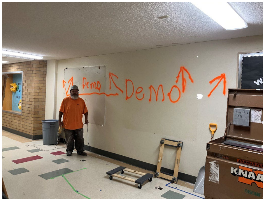
The "portal" connecting the elementary school to the new middle school was cut during the weekend.
