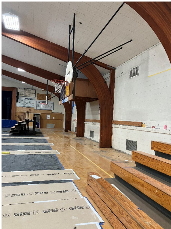
Demolition is complete for the KHS gym/cafeteria seismic project and the bracing/roofing/foundation enhancements are up and running.
