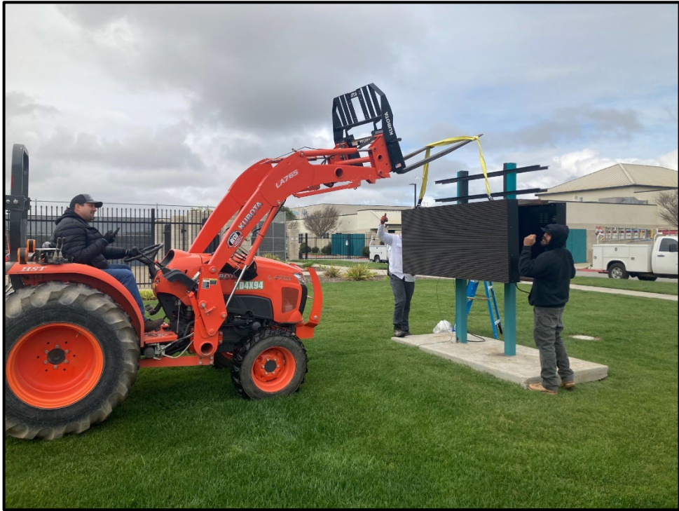
PVHS – Elias Camacho, Ernest Paz, and Thomas Harbold Completing the Marquee Installation
