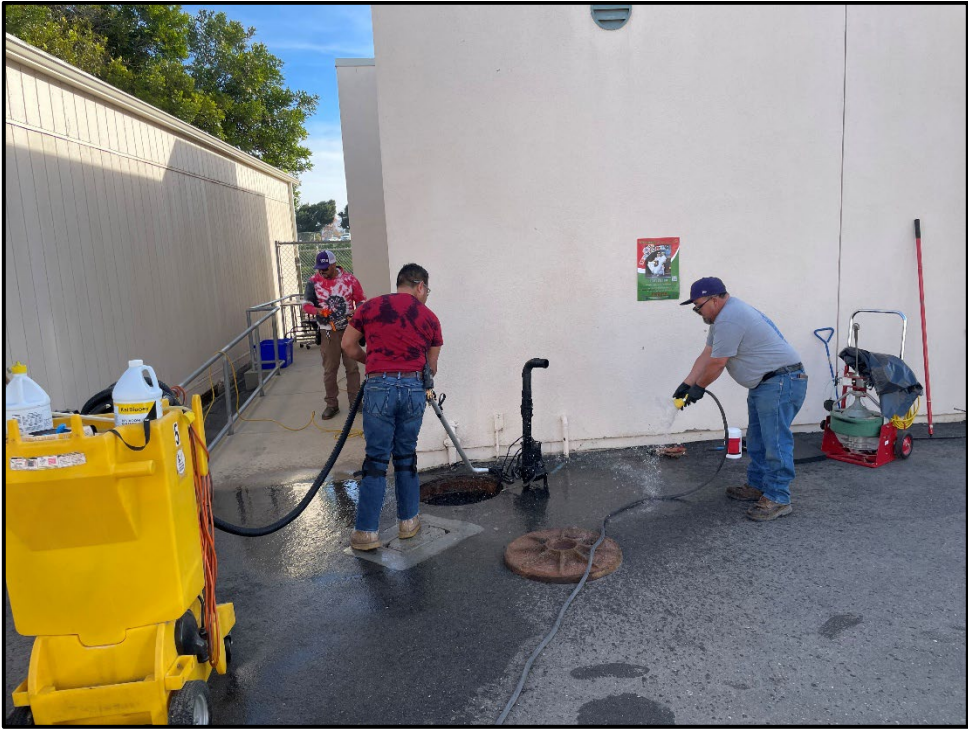
ERHS – Armando Gutierrez, Leo Avila, and Jesus Reyes Repairing a Broken Water Line
