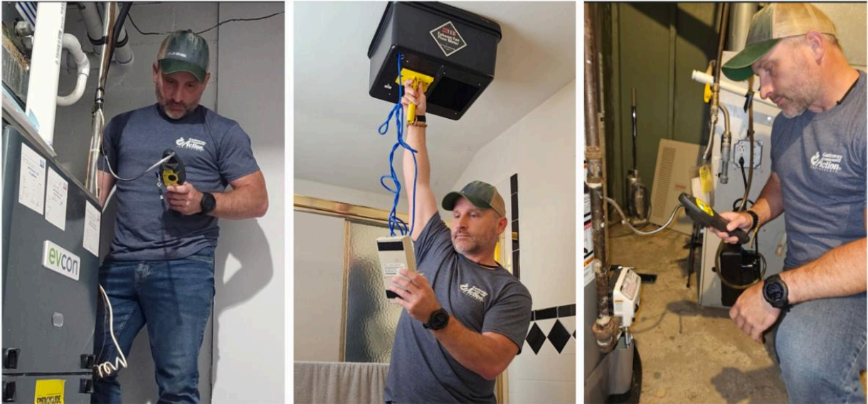
Senior Energy Auditor Eric Hasko conducts a series of home-safety and efficiency checks, including testing a water heater, evaluating a bathroom exhaust fan for proper airflow and performance, and inspecting the heating system to ensure there are no gas leaks.
