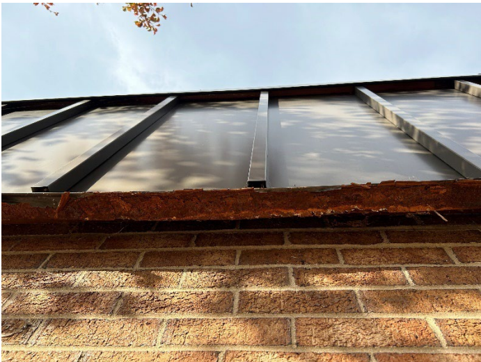
Failed metal standing seam panels
