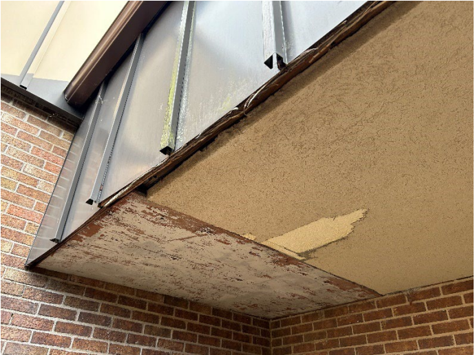
Failed metal standing seam panels & soffit
