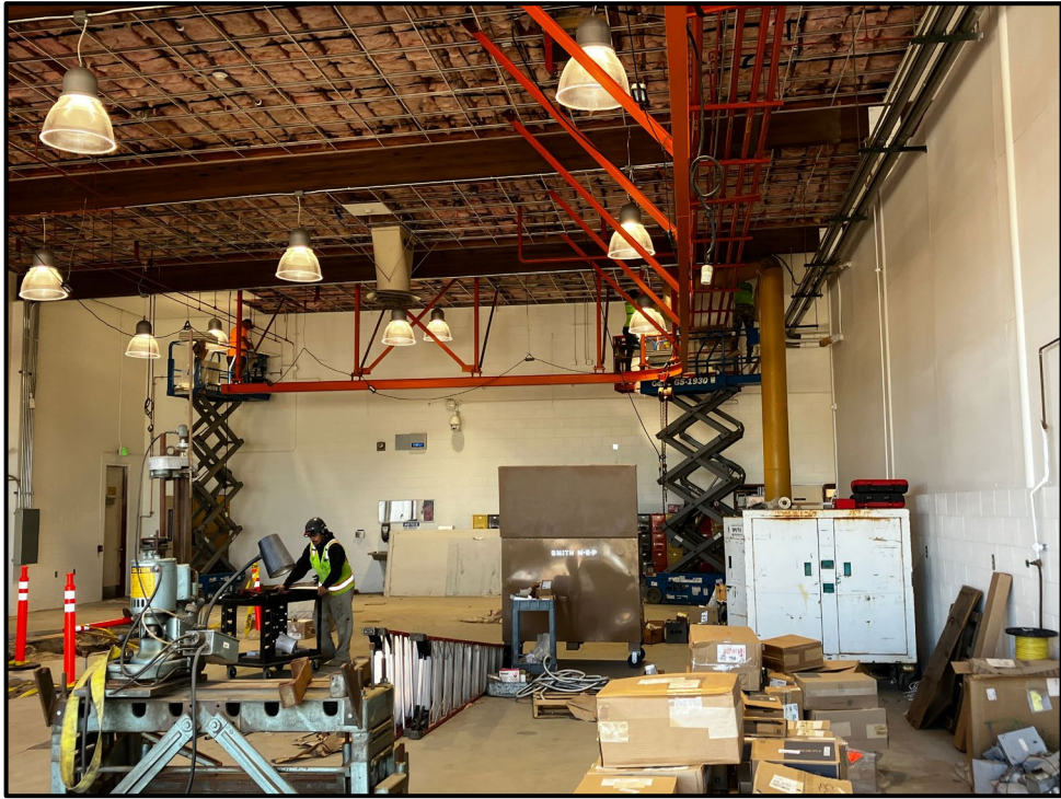
SMHS CTE Modernization – Installing Ceiling Tiles in the South Side of the Auto Shop
