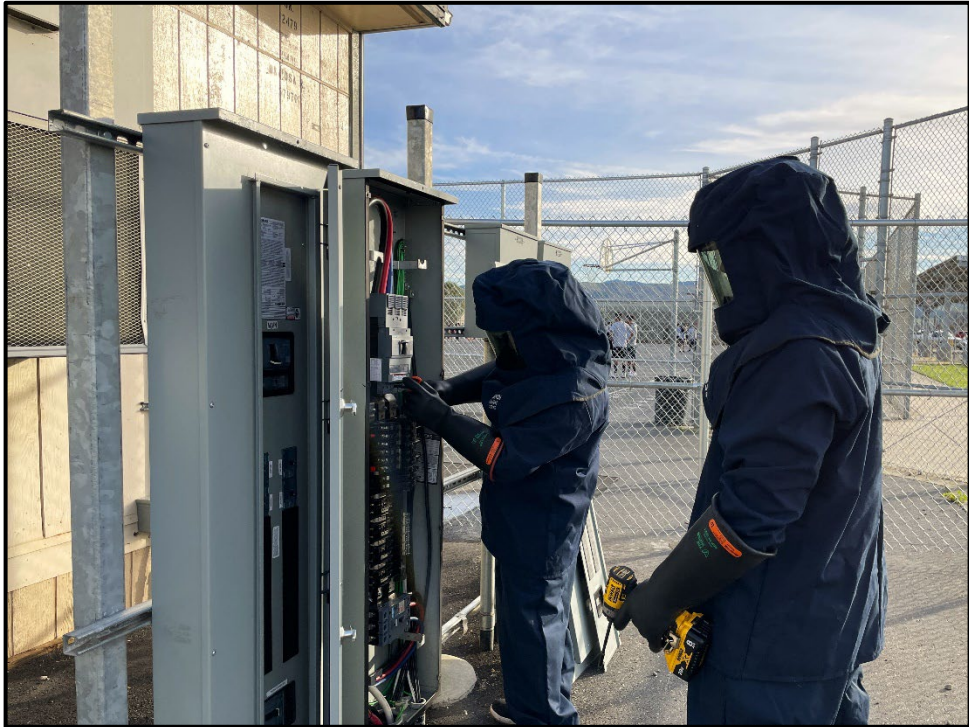
PVHS – Jesus Leon and Elias Camacho in Arc-Flash Gear Repairing Electrical Panel
