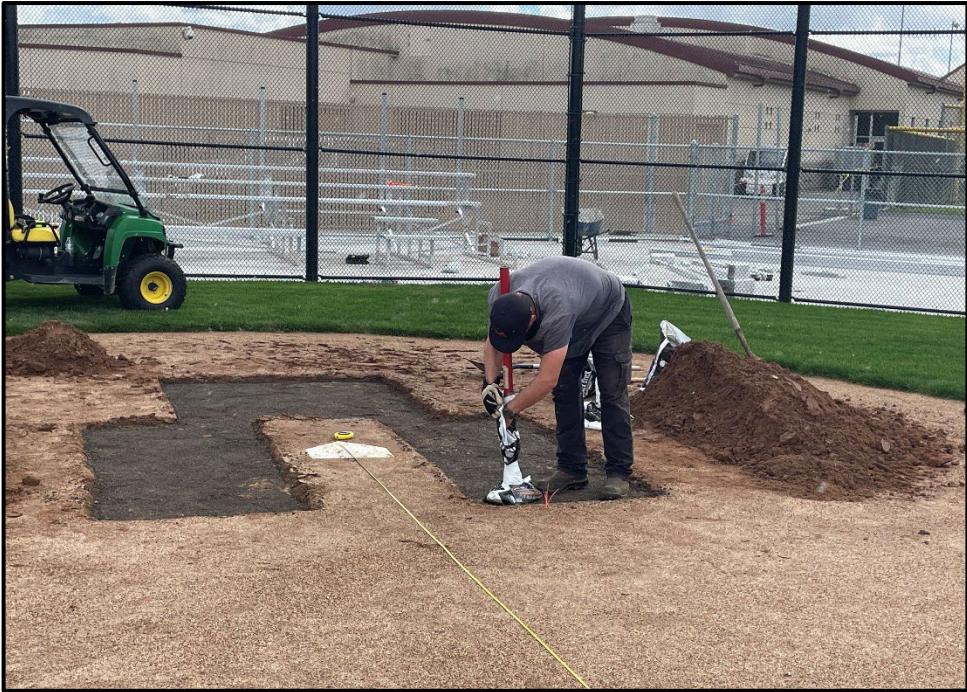
SMHS – Nick Canaan Setting Clay Base on the Newly Designed Softball Field
