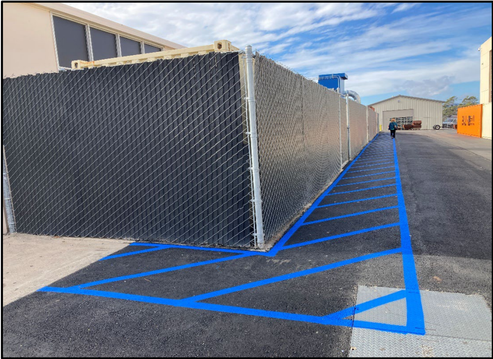
ERHS CTE Modernization – New ADA compliant walkway from the Welding Shop to the Gymnasium Patio is Installed
