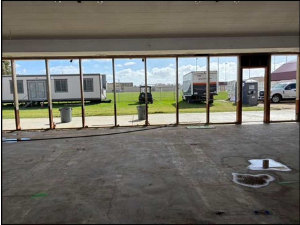
SMHS 37 Classroom – Demolition of Exterior Wall Where Nano Glass Wall Will be Installed
