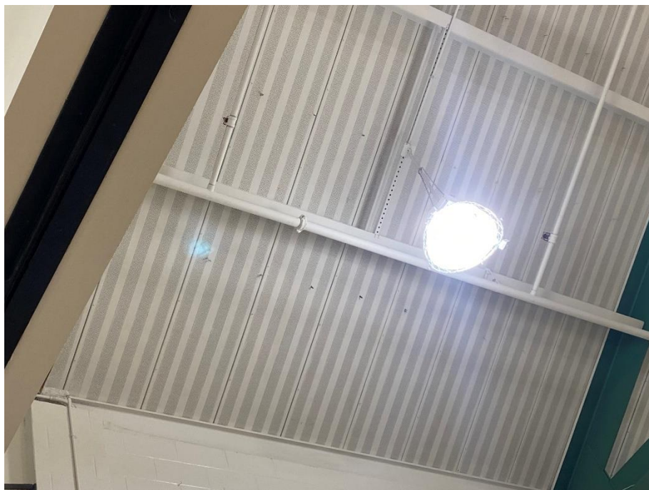
Photo 8: Inadequate clip spacing at eave
