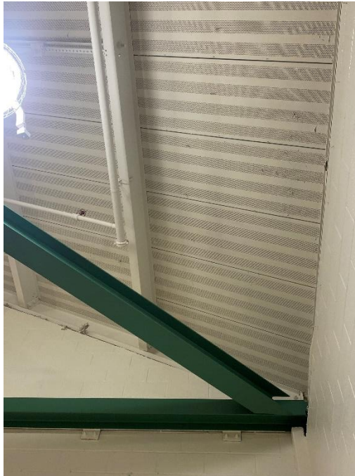
Photo 7: Inadequate clip spacing at corner
