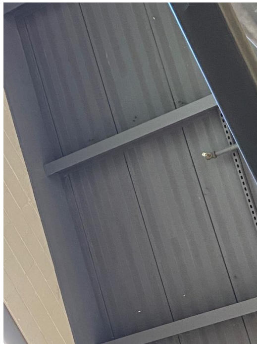
Photo 4: Excessive fastener spacing at gable end
