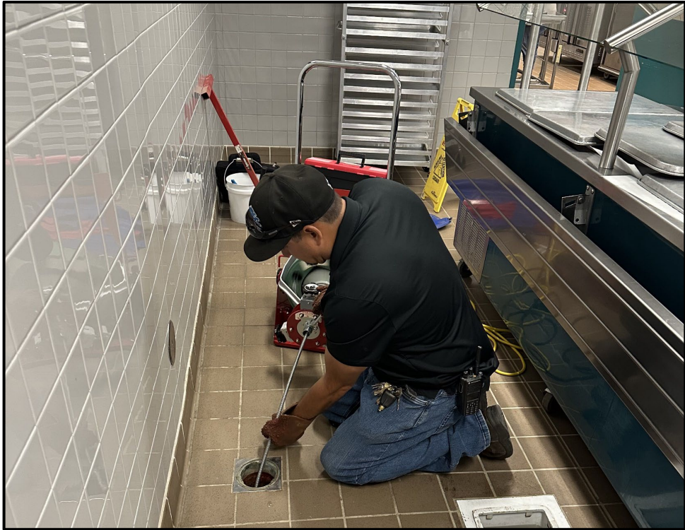
PVHS – Elias Camacho Cleaning the Drains in the Cafeteria Kitchen
