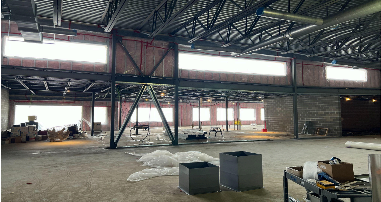
Work continues in the commons area on the north side of the new addition.
