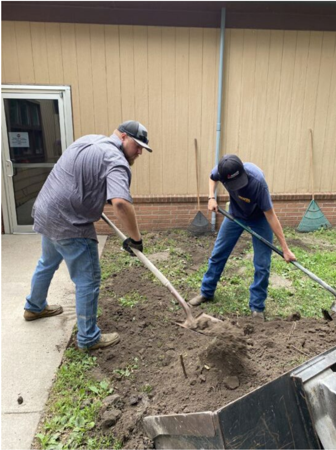
Curtis Heuermann, NC's new Director of Building, Grounds, & Transportation, leads the crew in work all across campus.
