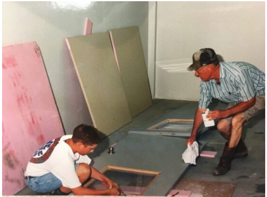
Clint Patrick (left, class of '00) helps Les McHargue prepare doors for installation.
