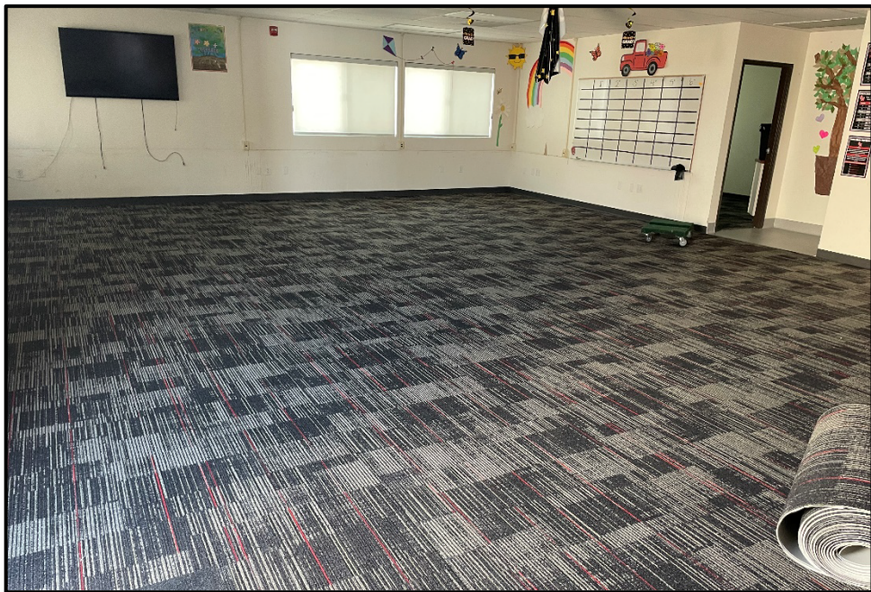
District Wide Carpet Installation – Carpet is Being Installed at SMHS, ERHS, PVHS, and the Support Services Center
