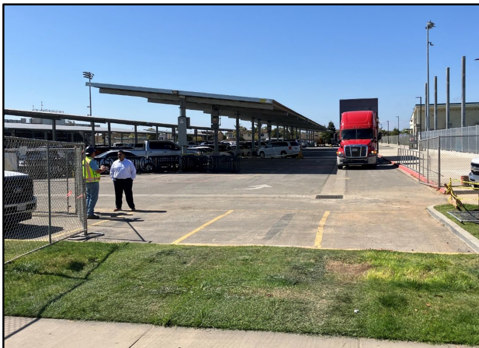
PVHS New Modular Classrooms – Antonio Garcia Observing the Building Section Crane Operation as another Section Rolls in.
