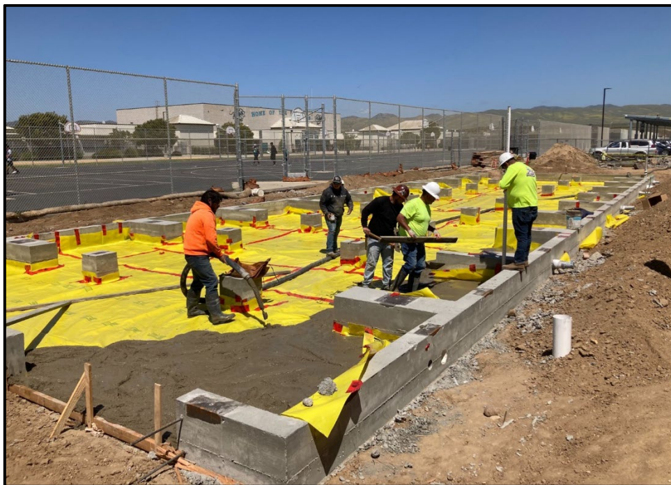
PVHS New Modular Classrooms – Concrete Slurry is poured to Prevent Weeds and Gopher Activity Under the Buildings
