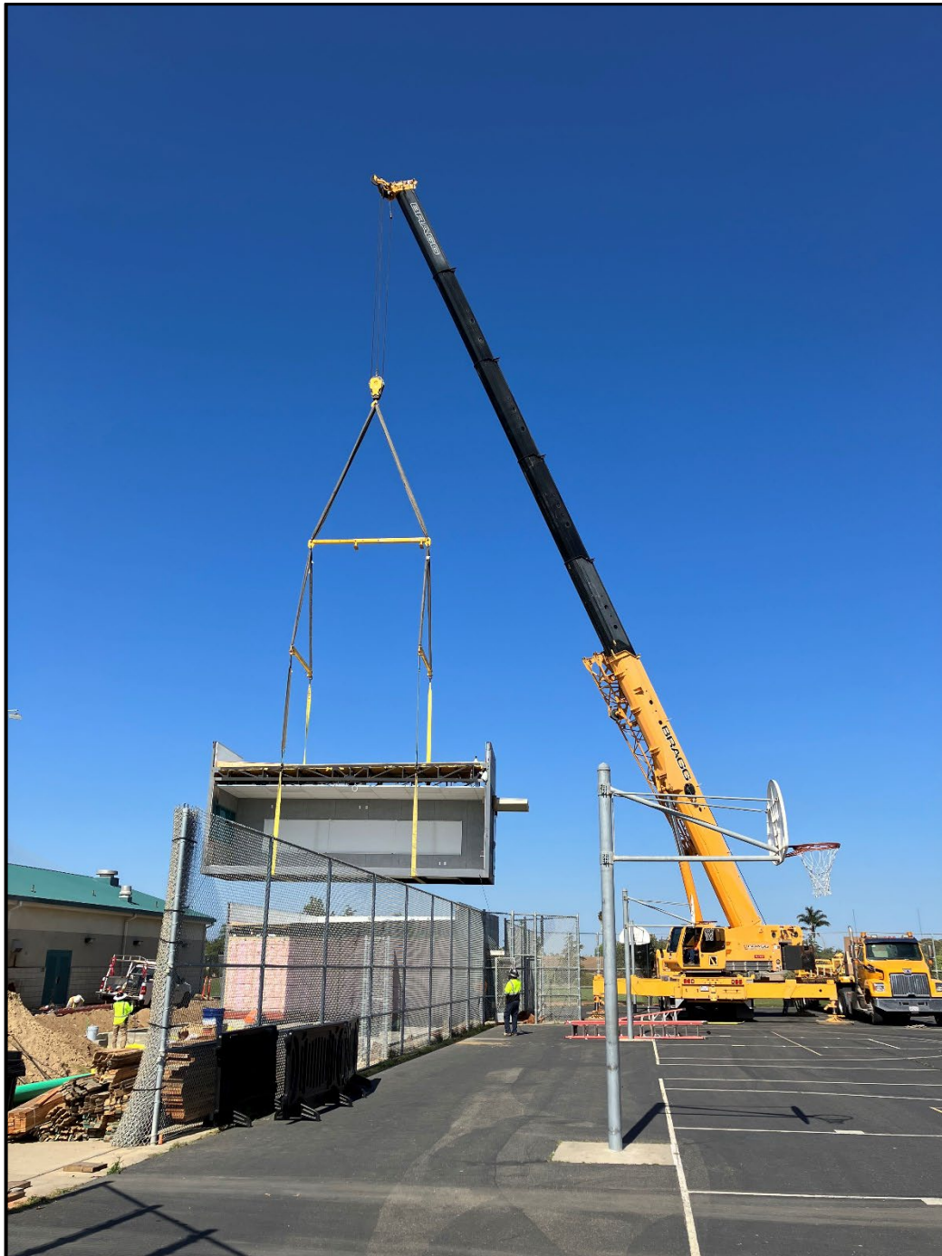
PVHS New Modular Classrooms – 140-Ton Crane Lifts the Building Sections and Sets them on the Foundation
