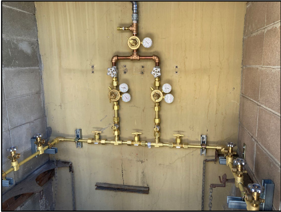
ERHS CTE Modernization – New Welding Gas Manifold Installed at the Welding Shop
