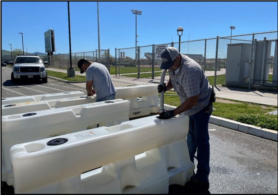
PVHS – Ricardo Eliserio and Elias Camacho Installing Delineators in the Student Parking Lot
