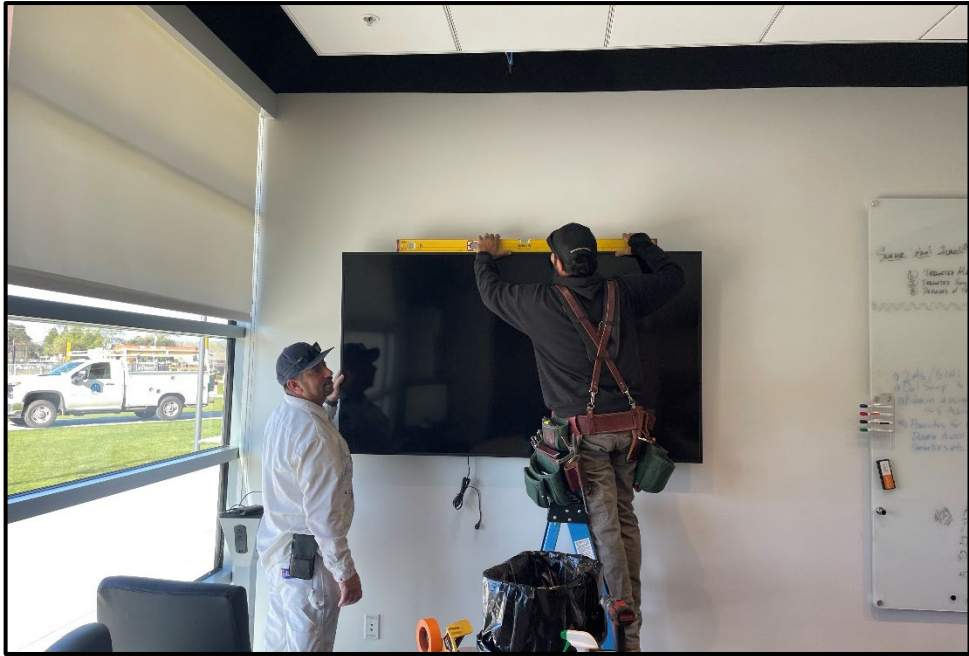
SMHS – Ernest Paz and Tom Harbold Installing a Monitor in the Principals Office
