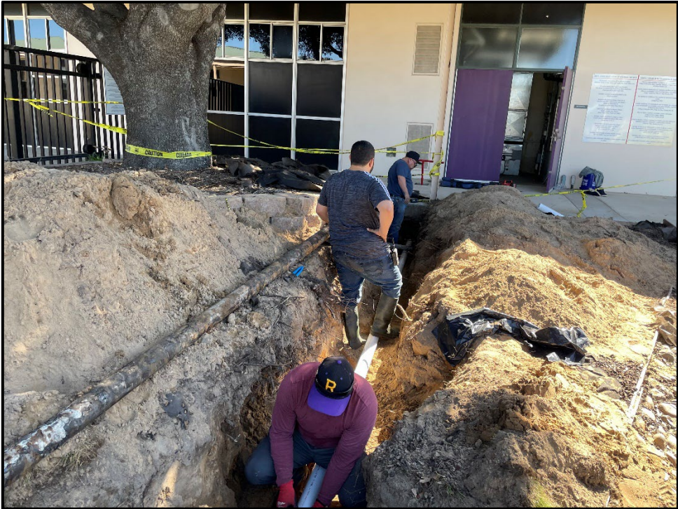
ERHS – Jesus Reyes, Eduardo Alvarez, and Joseph Campos Repairing a Mainline Water Leak
