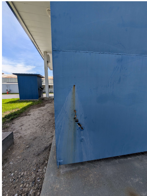
Exhibit 1-20: Fuel Storage Tank
