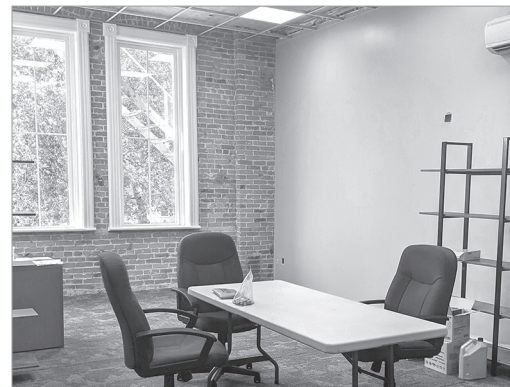
Room 11 in the Ad Building (the room directly across the hall from the front office) is in the midst of renovations and is already being used part-time as Superintendent Hekrdle's office. Once the renovation is done, new office furniture will be added.
