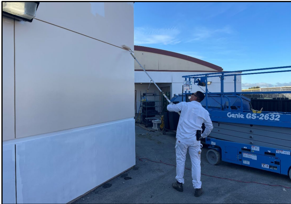
SMHS – Joel Amezcua Painting the Exterior of the Cafeteria MPR and Room 480
