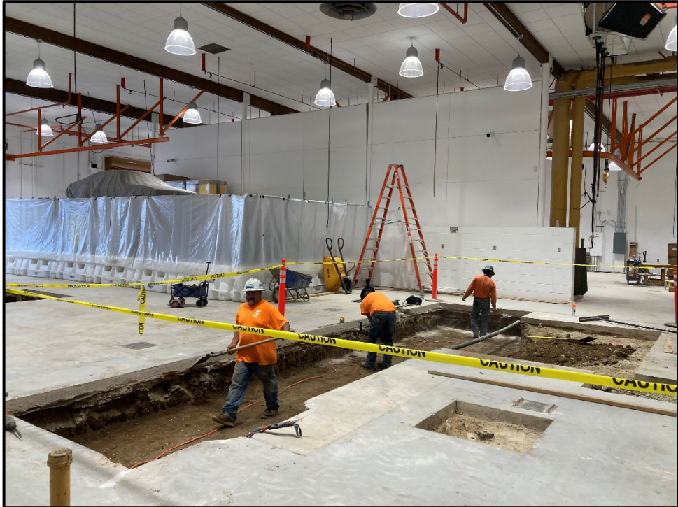
SMHS CTE Modernization – Auto Shop Concrete is Removed for the Lift Footing Installation
