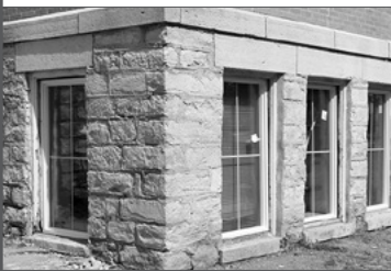
Window installation is progressing rapidly, with most of the basement-level windows being installed within the first week of July.
