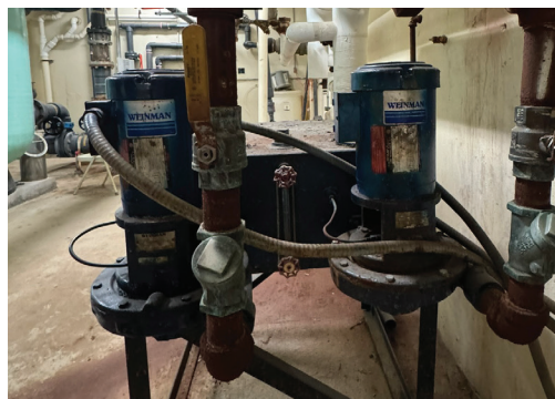
Aging pool mechanical equipment at the 6th-12th grade campus in need of replacement
