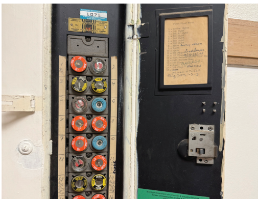
Fuse panel slated for replacement at the Washington Campus
