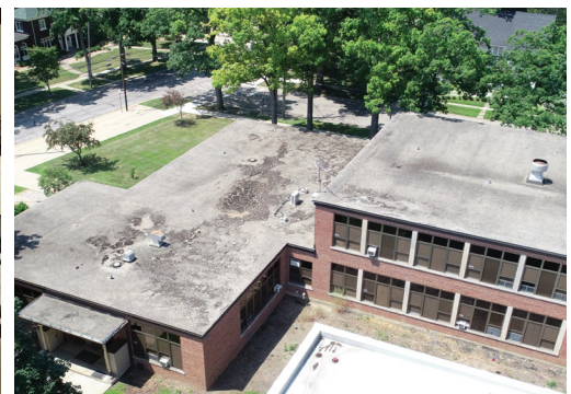
Roof at Central Elementary in need of replacement
