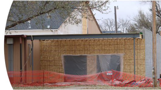
The new restrooms and entryway are being built onto the south side of the current gym building
