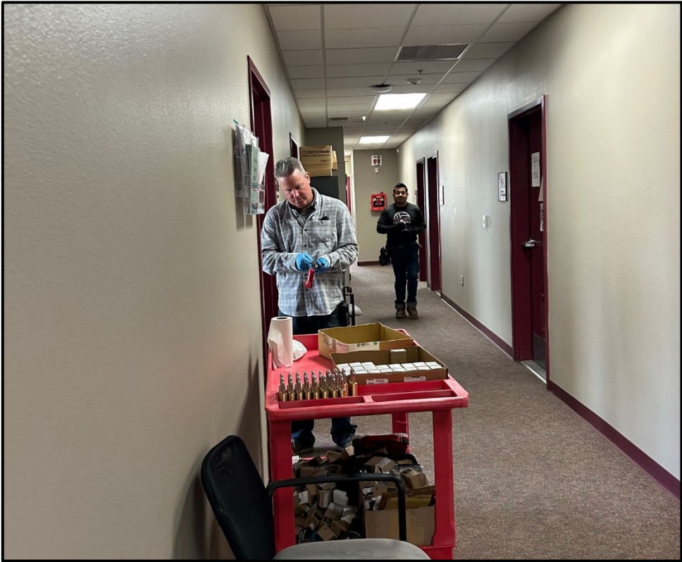
DHS – Dan Mather and Leo Avila Installing New Lock Cores Campus Wide
