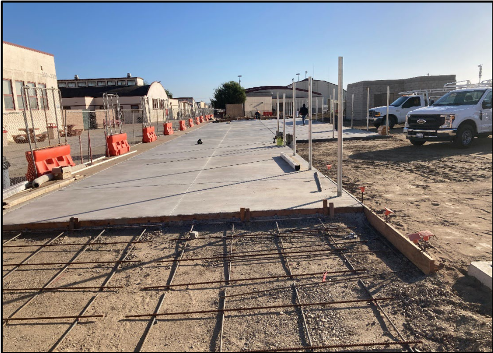
SMHS Reconstruction – Concrete Poured on the East Side of the New Softball Field
