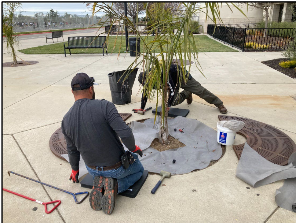
PVHS – Jose Gamino and Joseph Campos Installing Weed Barriers in Front of the Gymnasium
