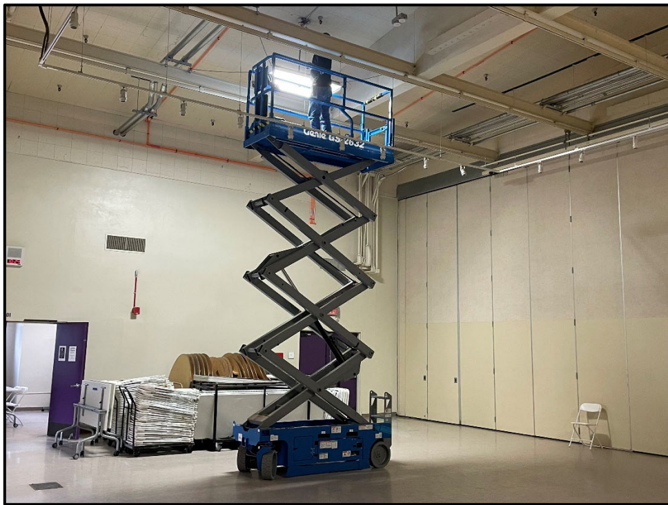
ERHS – Del Ward Installing Lighting and Motion Sensors on the Gymnasium Stage
