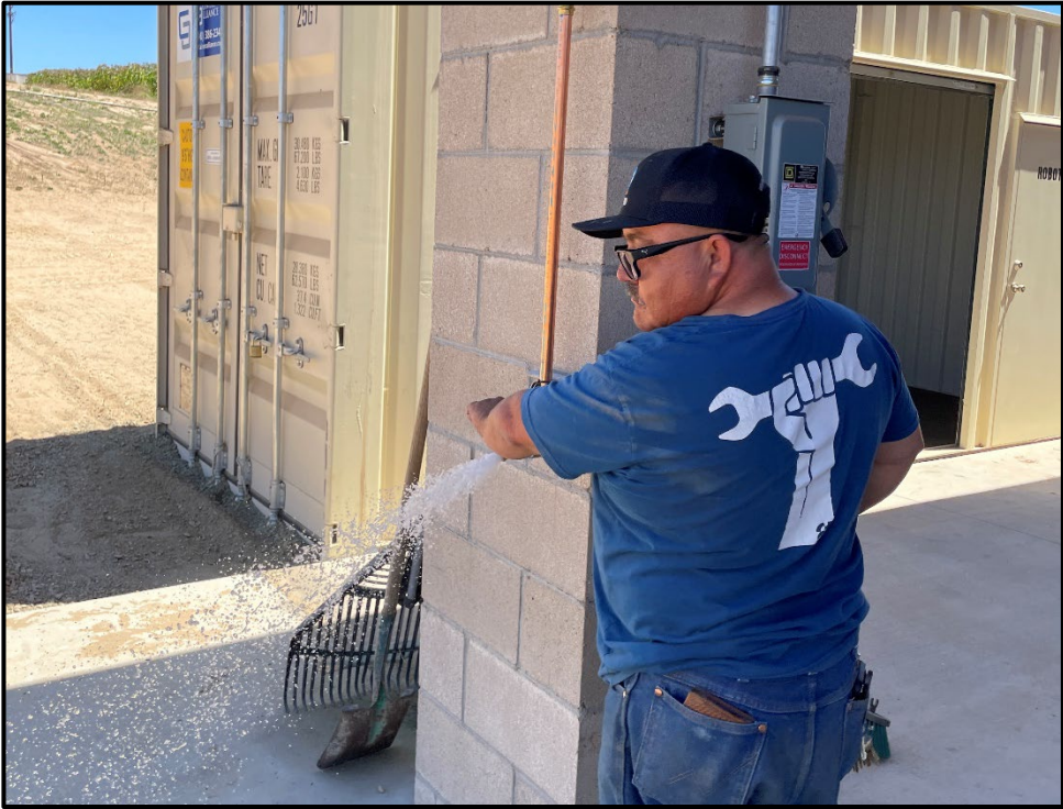
PVHS – Jesus Reyes Installing a Hose Bib Outside of the Culinary Arts Classroom
