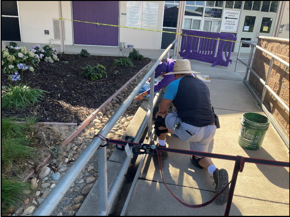
ERHS – Leo Avila and Armando Gutierrez Repairing the Handrail Outside of the Administration Building
