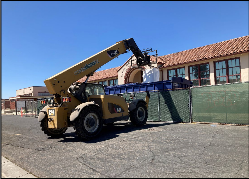
SMHS Admin to Classroom –Potentially Hazardous Materials are Being Removed and Disposed Of
